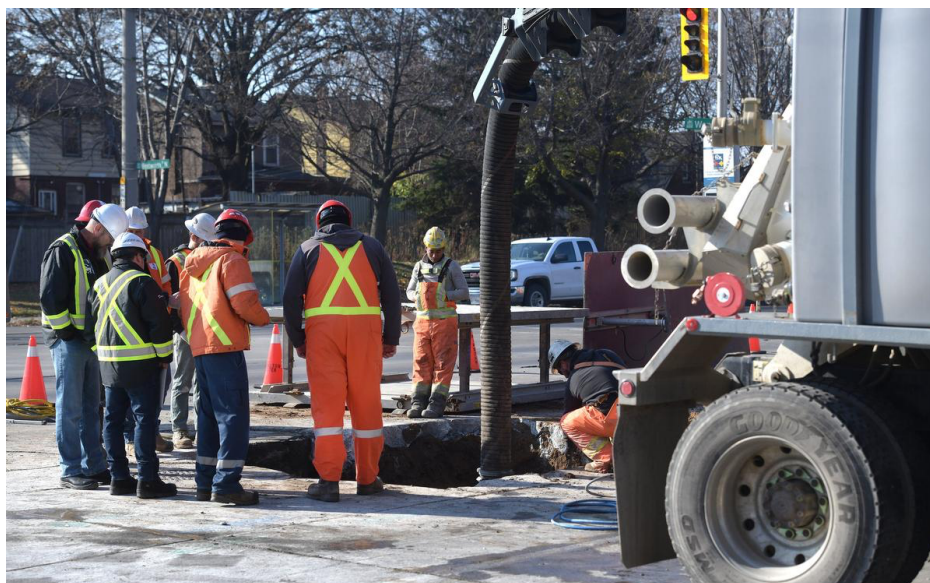
Figure 4: City crew working to repair 26-year-old misfitted sewer pipe near Burlington and Wentworth streets (The Spec)
